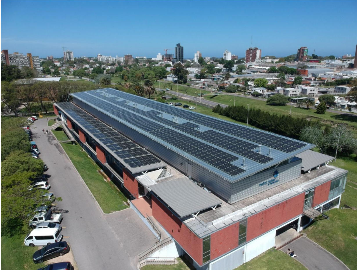
Roof with solar panels
